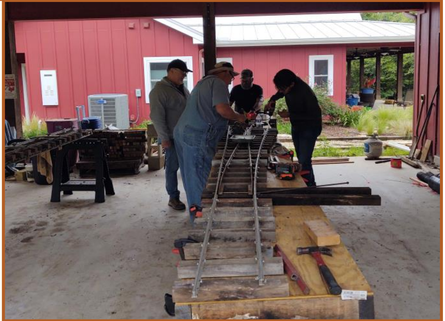
April 2023: Tim Boswell and Ken Rhodes take a break from the panel jig on the left to supervise John Oglesby and Jason Brownlee rebuilding a switch.
