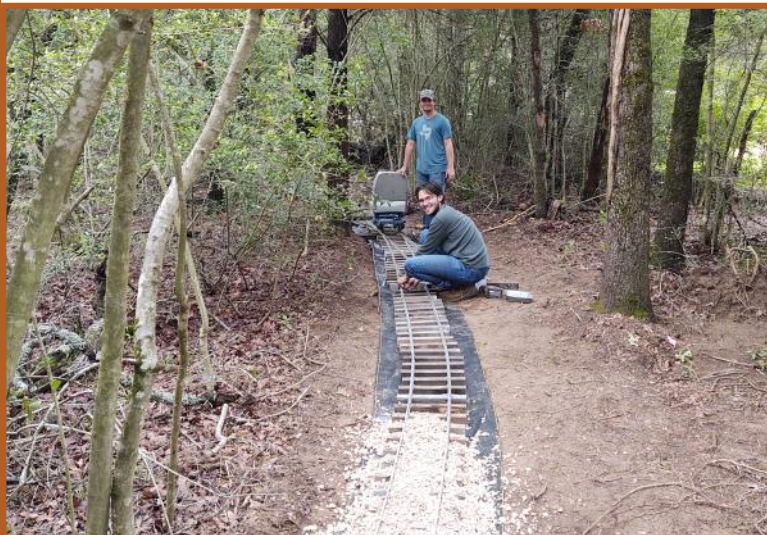
April 2023: Steven Tacconelly and Jason Brownlee laying track. This is the industrial area of Bexar which will have 3 tracks with a ground level turntable for engines to turn and run around.
